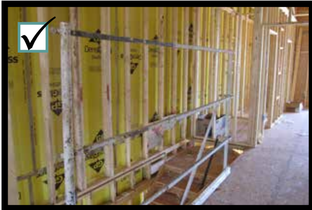
Erect guardrails around stairs.
